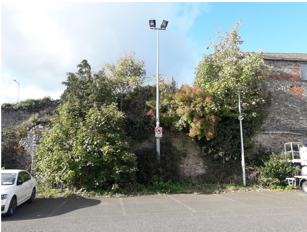
Photograph 9: Group 38. These self-seeded trees are growing on top of (or at the base of) the old stone wall. As with tree 12, the root systems are unlikely to fully develop, resulting in the failure of the trees, and the weakening of the wall.
